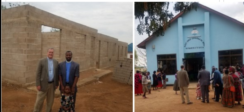
Nuru Lutheran Church at Kisesa, and their new children’s ministry building under construction. Jim Tino with Dixon and daughter Millcah.
